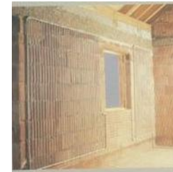
Chauffage surfaces murales
